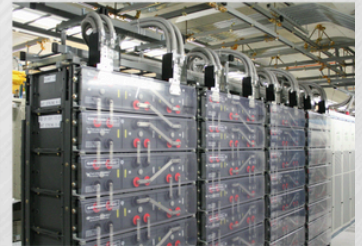
Telecom & Data Centres
