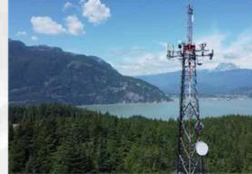
Telecom Base Station
